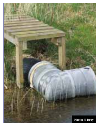
Fig 7: Right angled bend (& operator access platform)
