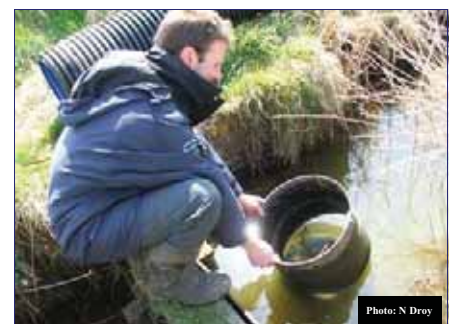
Fig 3: Adjustment of pipe control
